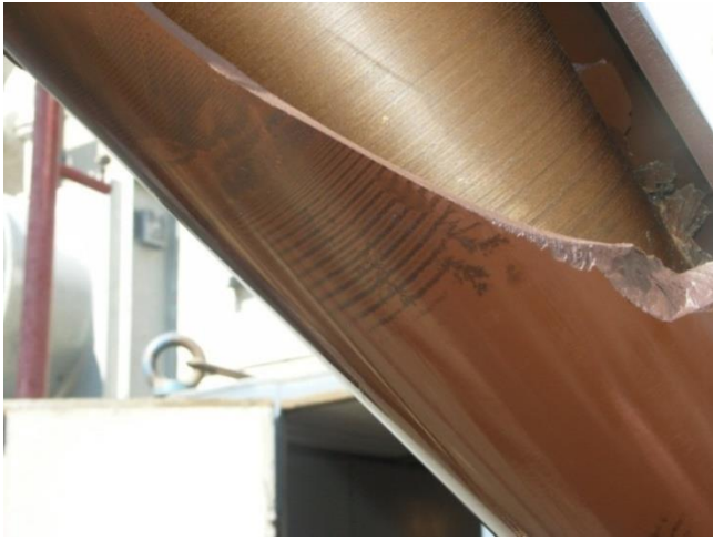
Fig. 2. The lower part of the 500 kV damaged bushing with traces of discharges on the external surface.
