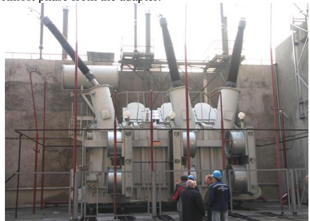
Fig. 1. Failure of a 500 kV block transformer after flashover of oil gap between bushing screen and adapter wall.
