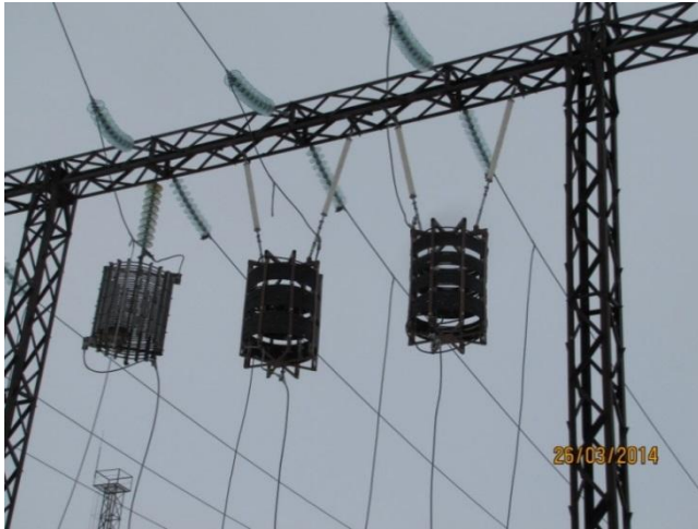
Fig. 2. On the left, the existing high-frequency line trap (stopper), in the center, and on the right is the mounted FDD. Substation Sugmutskaya, the Tyumen region, 110 kV.
